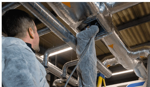
LEV System Cleaning
