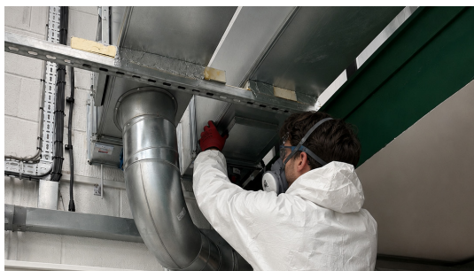
Laundry Extract Cleaning
