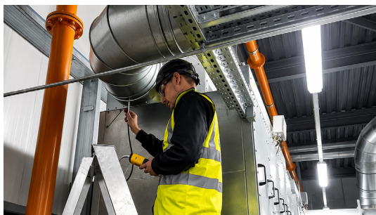
LEV System Testing
